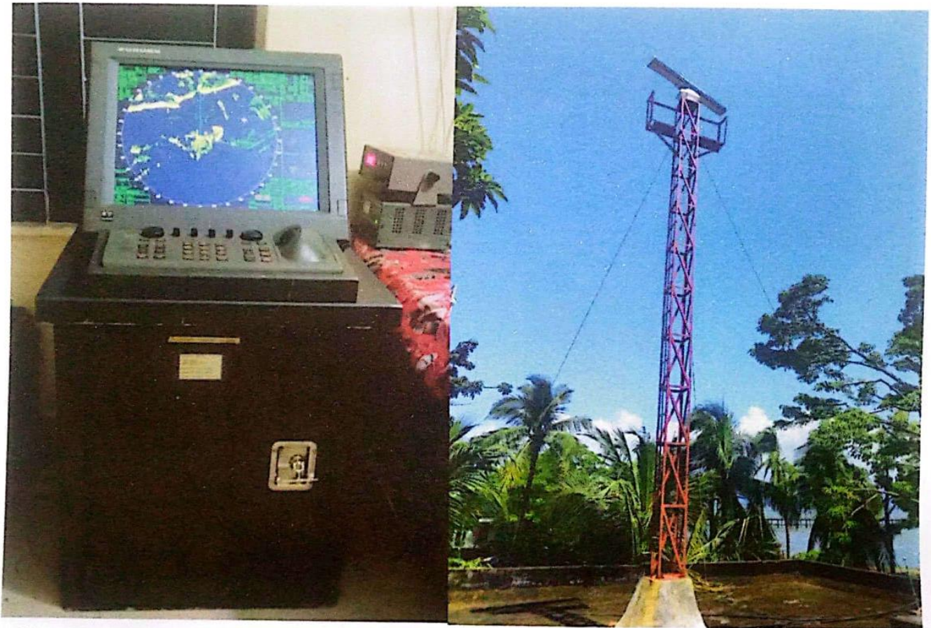
Surveillance RADAR of Shahporirdwip BOP
